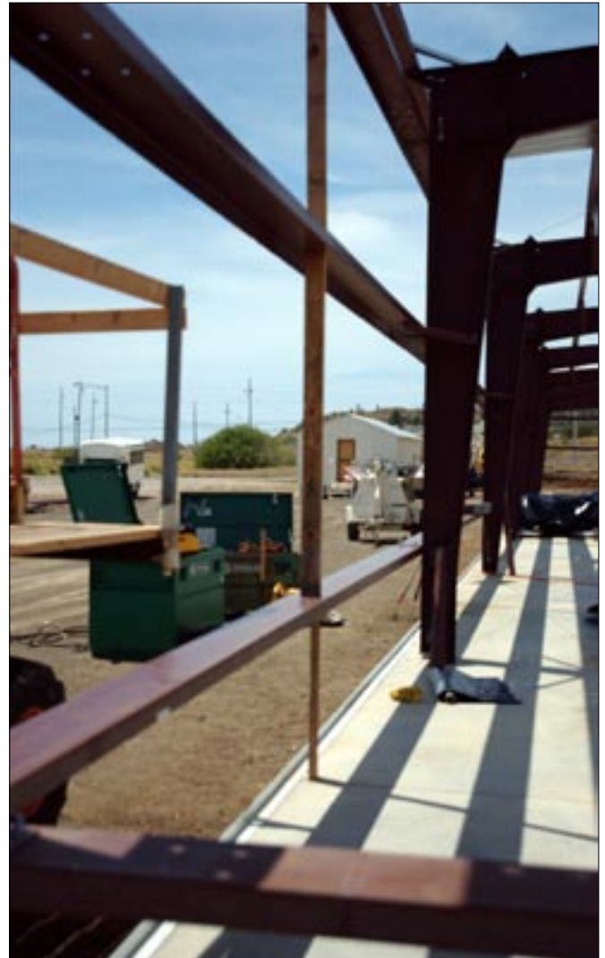
New construction on U.S. Naval Station Guantanamo's leeward side is part of a $16.5 million dollar contract to upgrade existing migrant operations facilities on the base. When completed, the camp will serve as a regional asset, providing shelter not only to economic and political asylum seekers, but also to victims of natural disasters.
