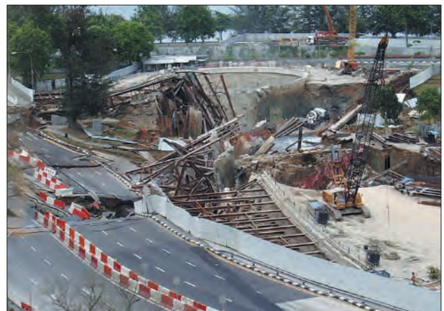
Abb. 1: Nicoll Highway Kollaps, Singapore
