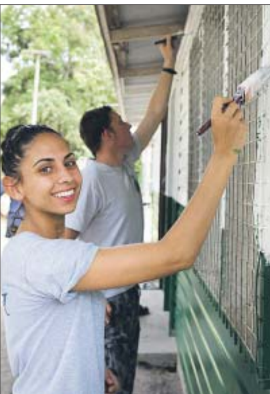
A NEW LOOK: ABMT Jessica Kelly joins fellow HMAS Gascoyne personnel in giving their time to paint classroom buildings at the Raluana Community School in Papua New Guinea. Photo: ABIS Sarah Williams
