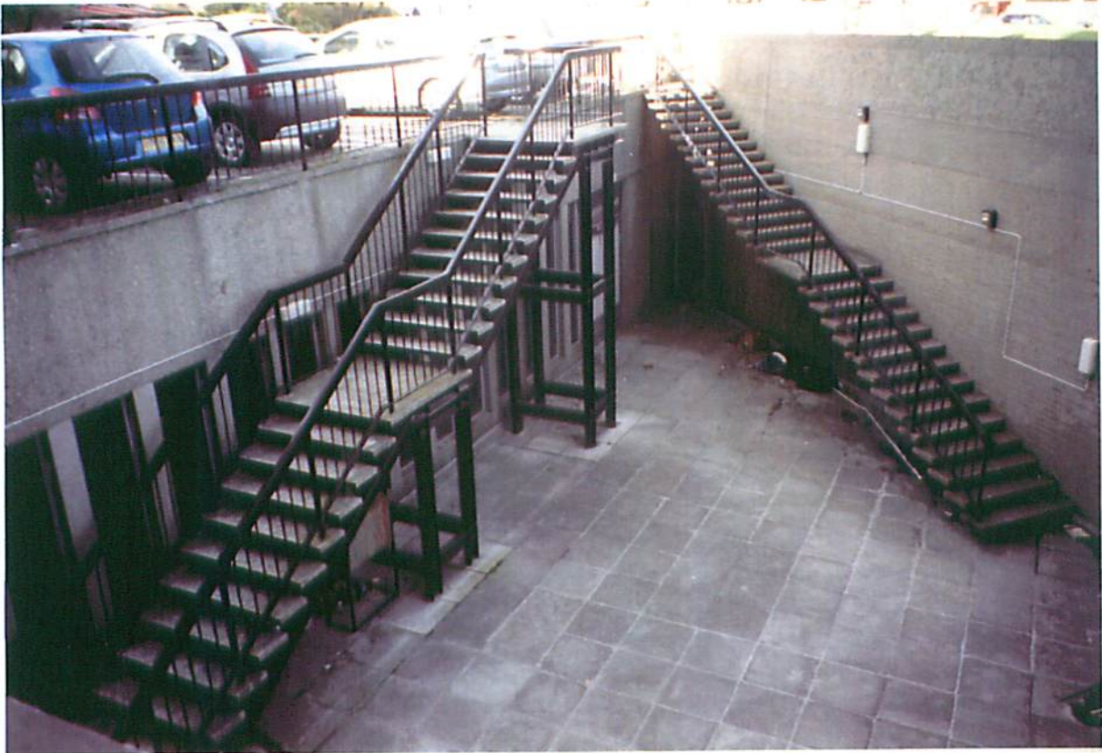
Original cantilevered concrete stair (right) and later steel addition to lower courtyard.
