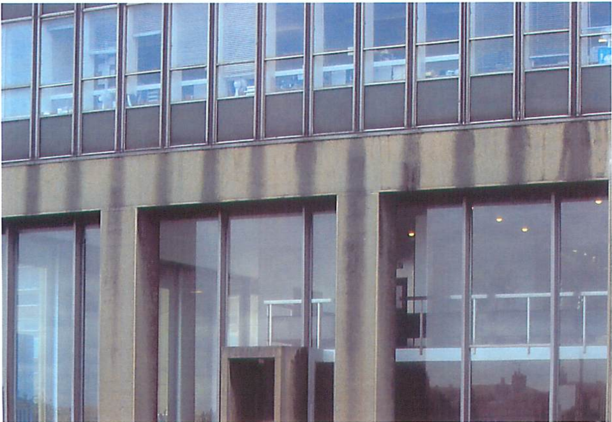
Detail of double height glass screen (rear) with later half-sized-replacement (right). Note also staining pattern on concrete fascia
