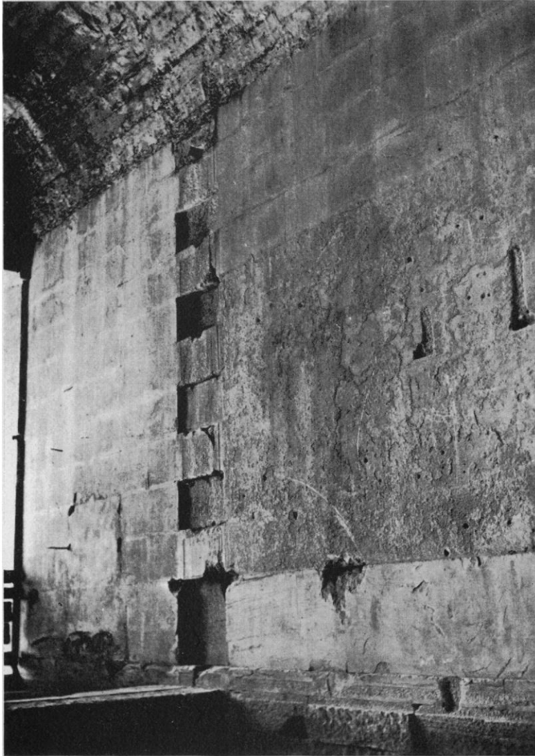
Fig. 31. South Wall of Cella at Junction with East Cross-Wall, Showing Mediaeval Plaster
