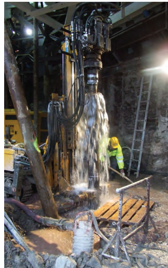
Wassara DTH water-powered drills and Grindex dewatering pumps are being used across the Citybanan project in Stockholm, Sweden
