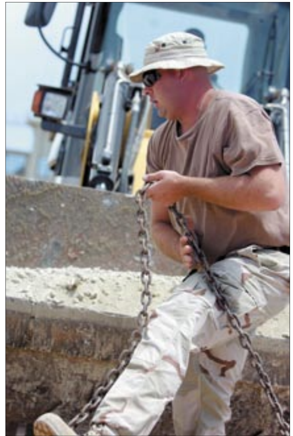
"Dirt boys" from the 474th Expeditionary Civil Engineering Squadron prepare to lay a permanent foundation for Guantanamo Bay, Cuba's new military commissions courtroom expected to be completed early next year. Using plattes developed by the 883rd Red Horse team, the 474th broke ground on the project Sept. 11. (Photo by Army Sgt. Sarah Stannard)
