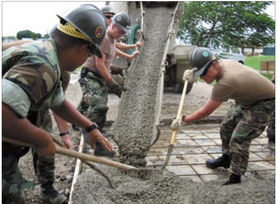
Seabees of the Fighting Forty repair a damaged section at the Leeward Airport on Thursday, Oct. 11. (Photo by Navy Seaman Kenneth Johnson)
