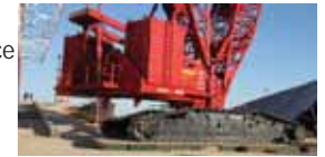
emtek mats providing a stable base allowing a 160t lift to be completed safely
