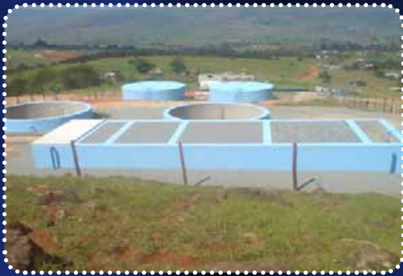
7. Lamgabhi water project treatment works
