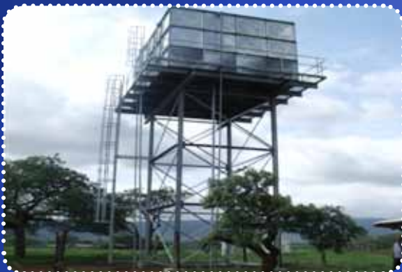
5. Becker elevated steel panel reservoirs at ndzevane rural water supply scheme
