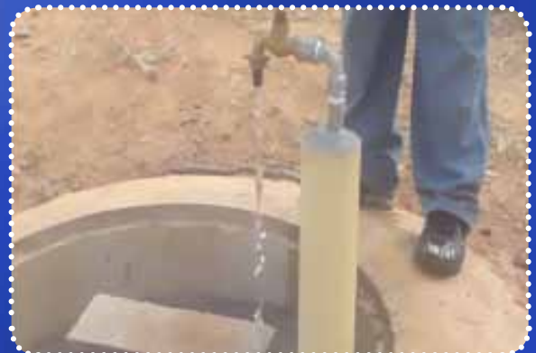
6. Stand pipe (siphofaneni umzabalazo wabomake water project)
