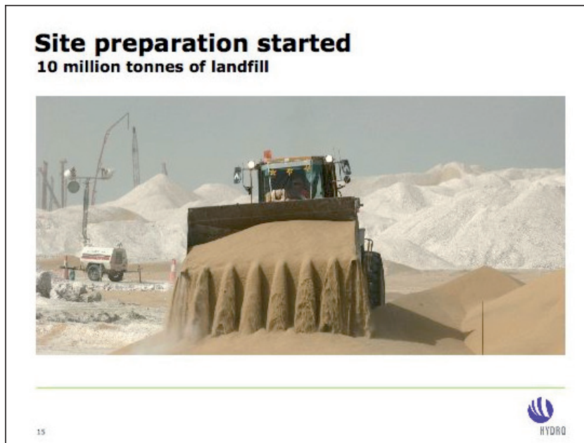
Figure 23. Challenges with sand in Qatar (Source: Tom Røtjer, Executive Vice President and Head of Projects, Capital Markets Day, 09.09.07)
