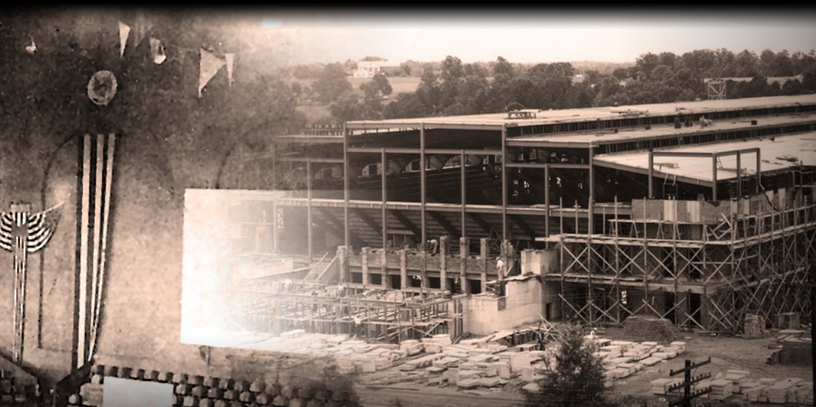
Construction began on Reynolds Coliseum in 1943, but was delayed many times during World War II.
