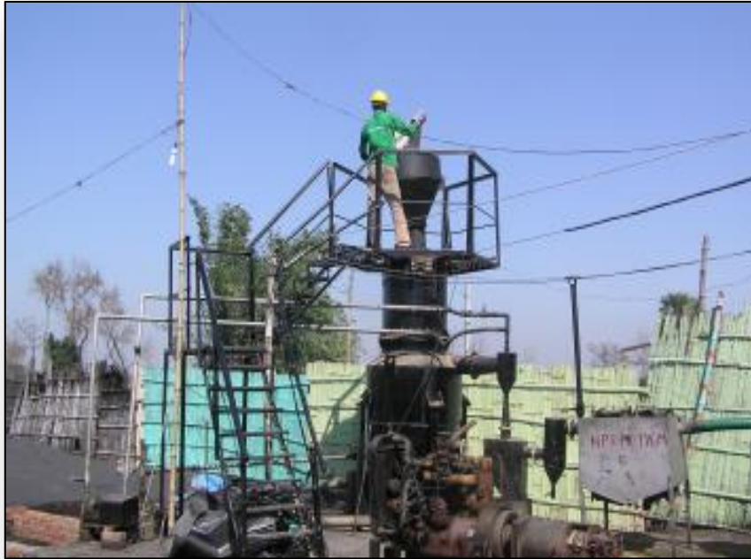
Filling a gasifier plant with rice husk, Tamkuha, Bihar.
