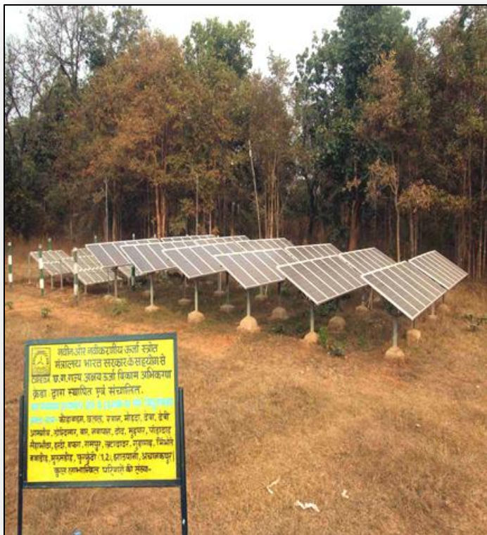
Solar PV power plant.
