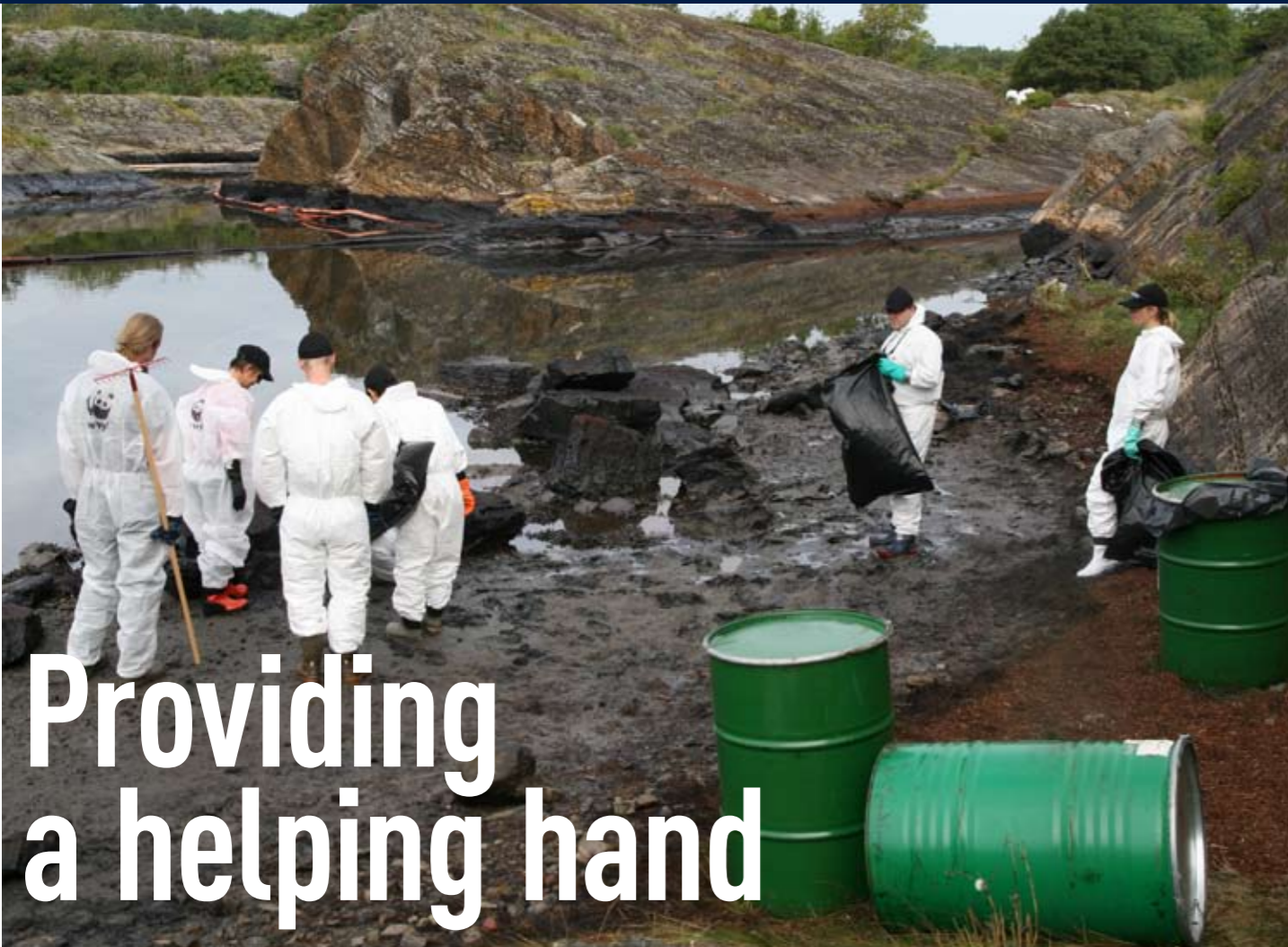
OIL EVERYWHERE: It was a sorry sight which met the volunteers who arrived to clean up after Full City's grounding off the coast of Norway.
