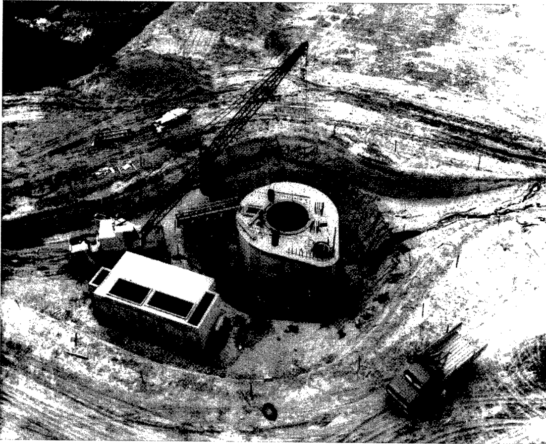
A Minuteman silo near Ellsworth AFB, South Dakota nears completion in June 1962. The rectangular launch facility support building is to the left of the silo.
