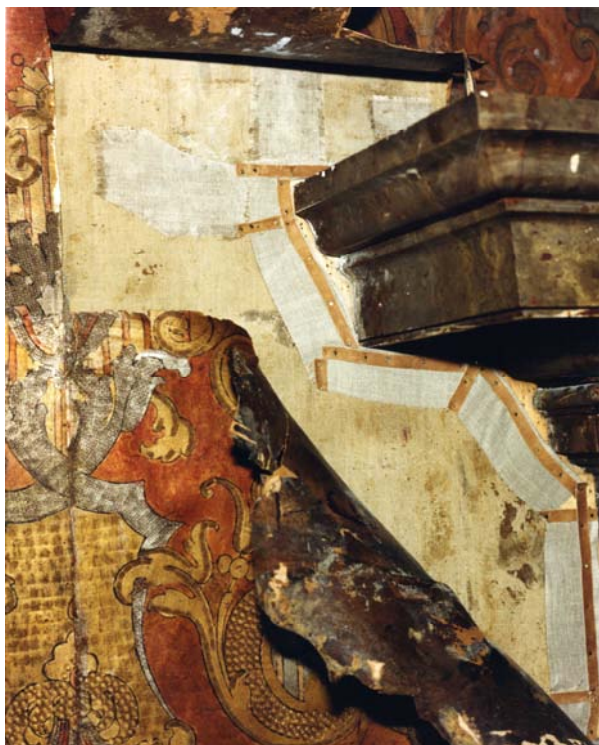
Fig. 7. Fixing the linen canvas to the wooden frames attached to the wall – leather strips protect the edges of the canvas against potential damages by the nails.
