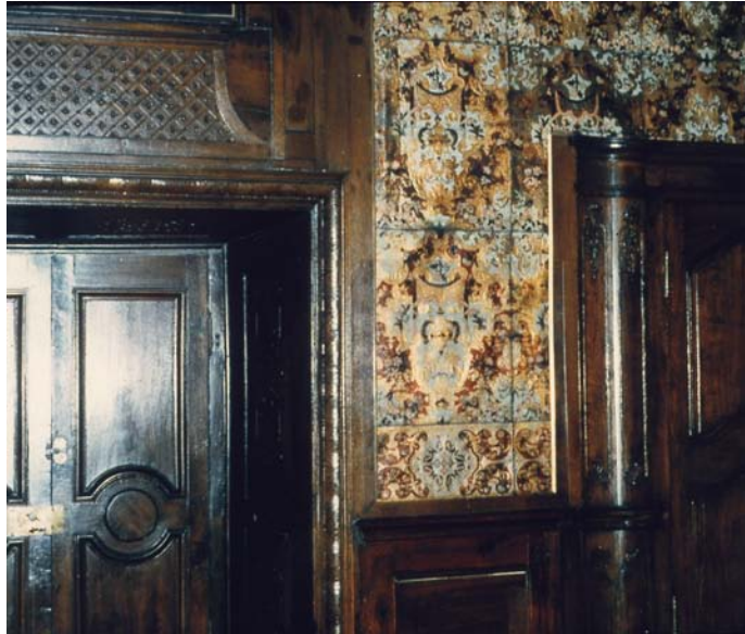
Fig. 1. Gilt leather in Dyck castle. Section with the test square before treatment. On the left hand side there are a large dark oil stains on the wooden panelling.
