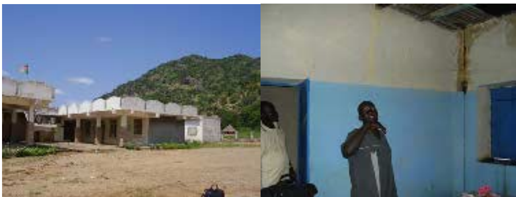
Kurmuk Town Hall/Civil Service Headquarters; and SRRC office in Kurmuk with leaking roof
