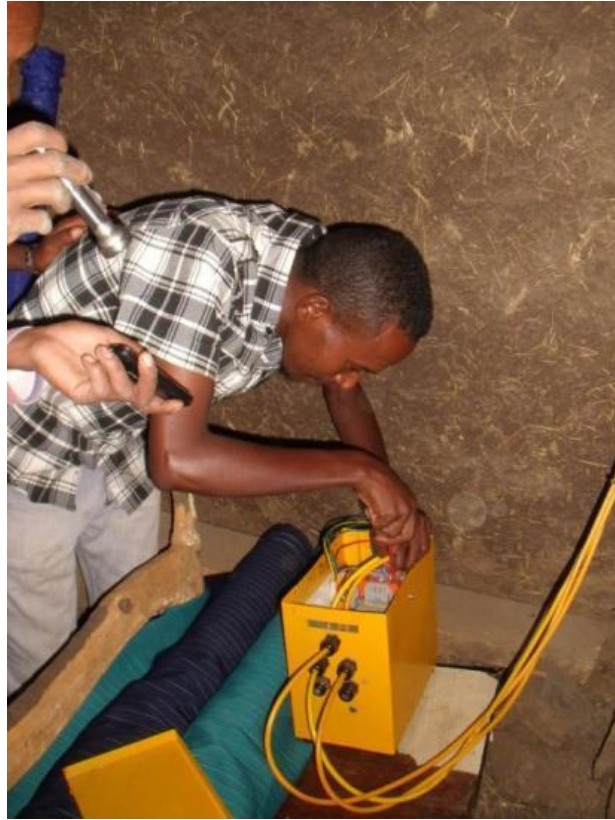
Picture 12: The team from the Solar Center in Rema repairs the power box of one SHS.
