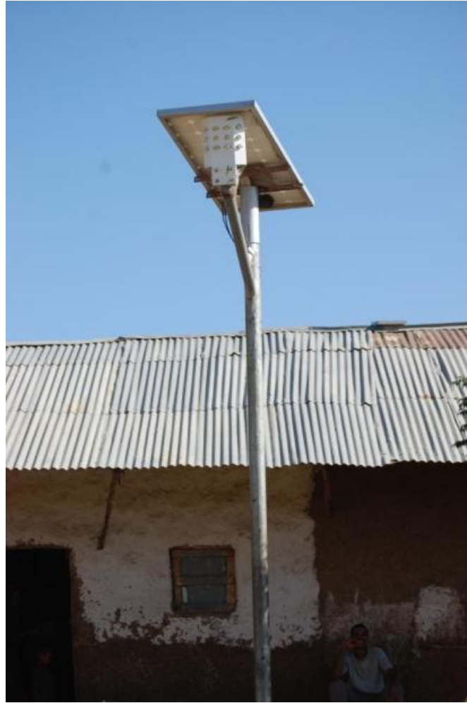
Picture 16: Solar street light at day...
