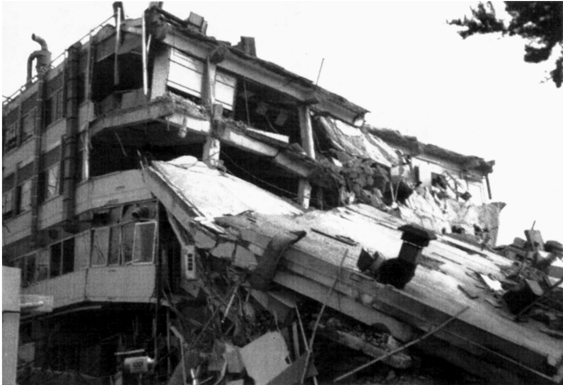
Fig. 12. Collapse of a concrete-frame pharmaceutical factory wing (damage degree 5) at Adames.
