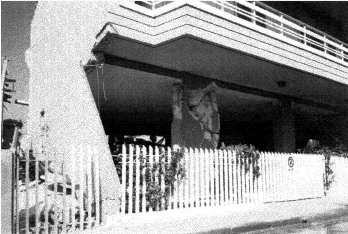
Fig. 5. Reinforced concrete column failure of a single-story building with damage degree 4 in Ano Liosia.
