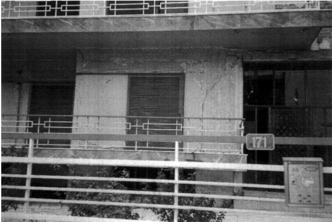
Fig. 11. Column failure of a reinforced concrete frame structure with damage degree 4 in Menidi.
