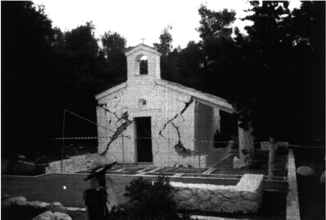
Fig. 7. Severe damage (Fourth degree) in a simple stone masonry church at Thrakomakedones area.
