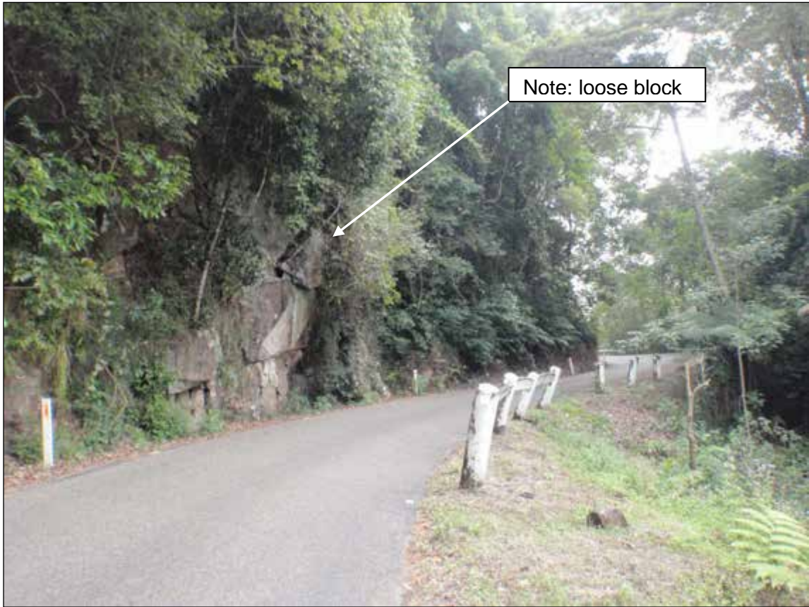
Photograph 12: Typical road cutting through bedrock on Paluma Road. Note the loose block that has the potential to fall onto road shoulder.
