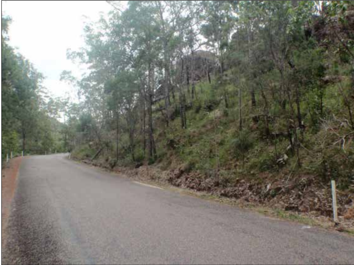
Photograph 14: Typical sloping ground above Paluma Road. Note the loose boulders on the slope that have the potential to cause rock roll.
