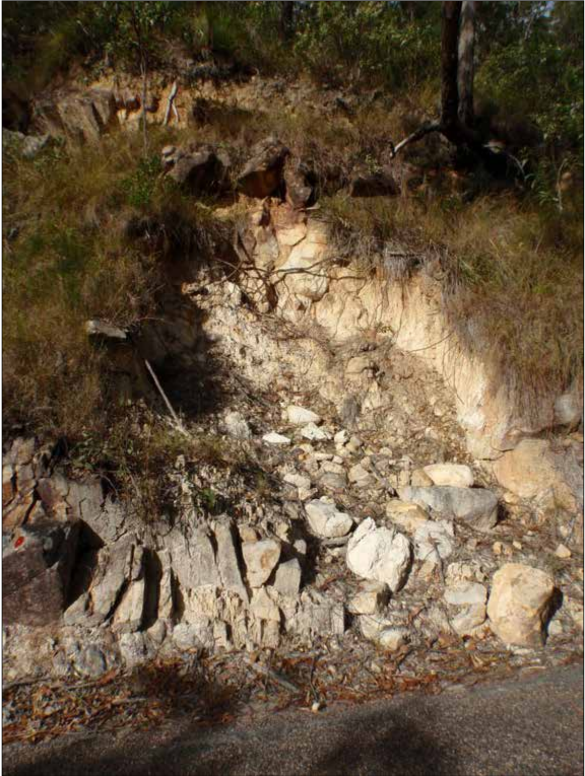
Photograph 5: Example of shallow slumping landslide.
