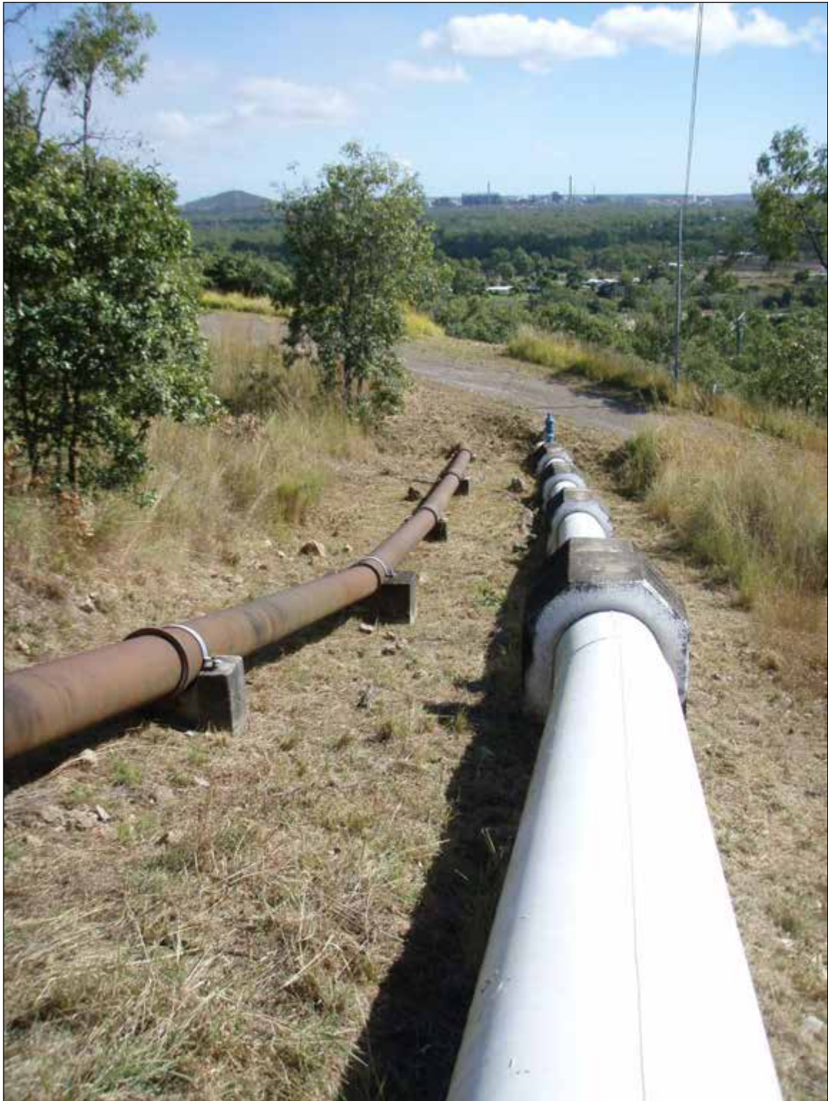
Photograph 11: Pipeline infrastructure on sloping ground at Jensen. Note small boulders that have rolled into pipeline corridor.
