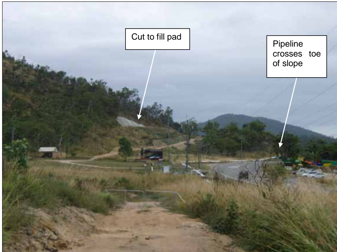
Photograph 15: View of Bruce Highway at Rollingstone looking north. Note that road and pipeline are generally removed from slope. Pipeline crosses toe of slope in right hand side of this photo. Note cut to fill pad on sloping ground (shotcreted) understood to be for future pylon construction.
