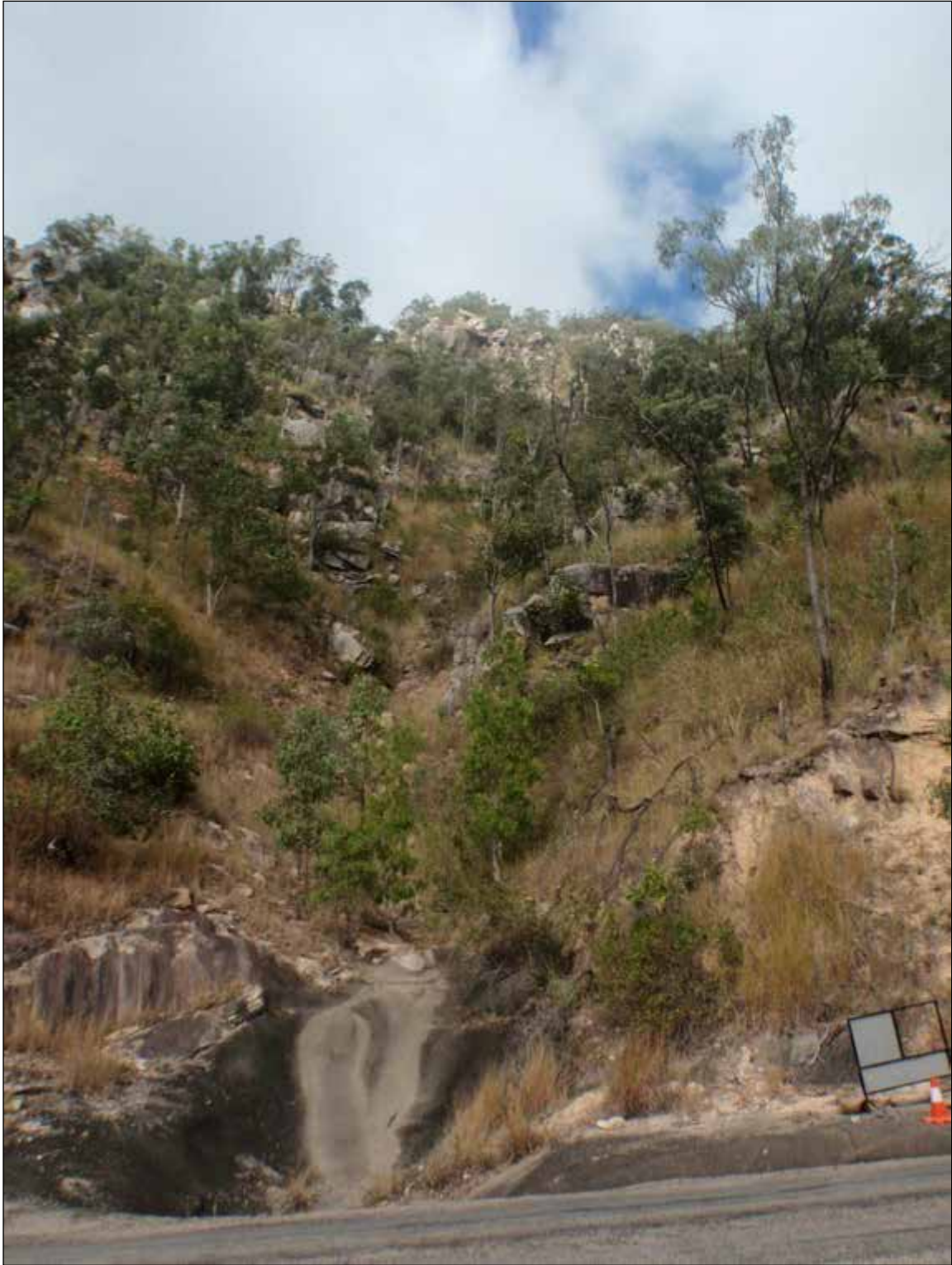
Photograph 16: View of steep gully above Hervey Range Road. Note some loose sediment and debris in gully base, may be susceptible to debris flow/ torrent.
