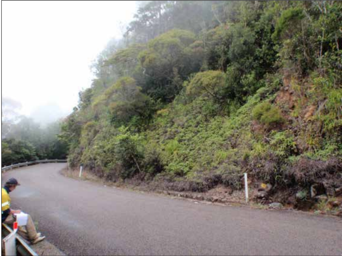
Photograph 13: Typical road cutting into base of slope on Paluma Road. Note the new vegetation that indicates previous slumping activity (slip scarp is visible on right hand side of slump).
