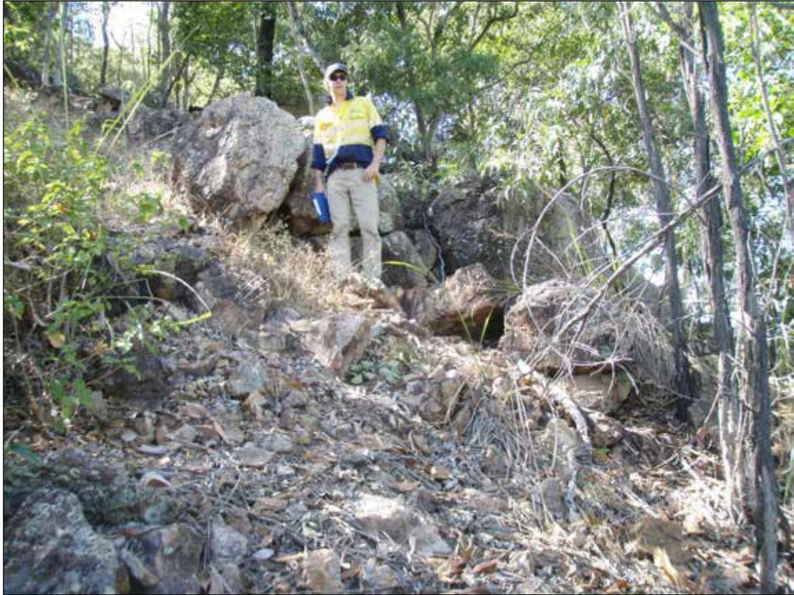
Photograph 6: Example of potential rock roll source.
