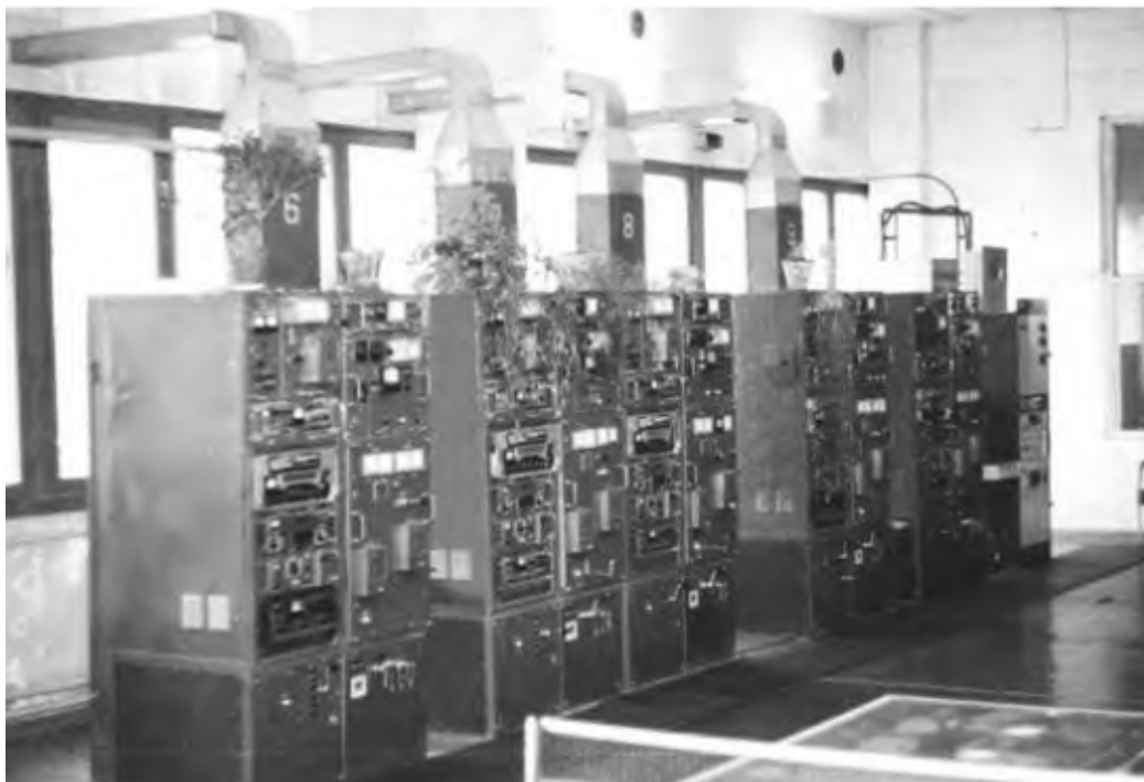
2.5/5 kW SW communications radio transmitters "Viaz-M2" at the local radio jammer near Panevėžys in Lithuania.
