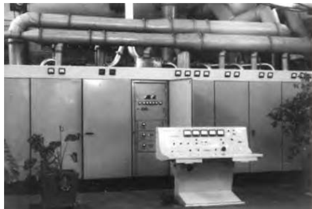
500 kW MW transmitter "Vikhr" was a reserve unit for jamming at Sitkūnai radio station in Lithuania.
