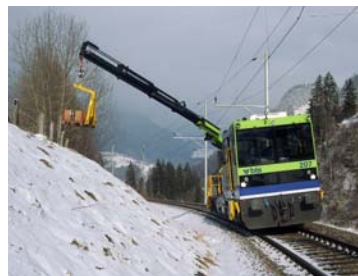
Maintenance vehicle Tm 235
