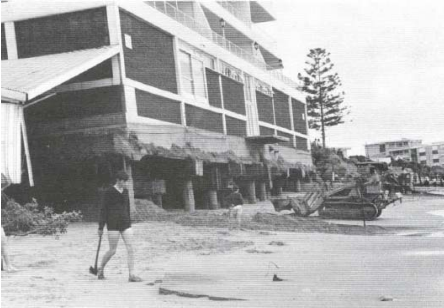
Exposure of 'Flight Deck' foundations as a result of 1967 storms
