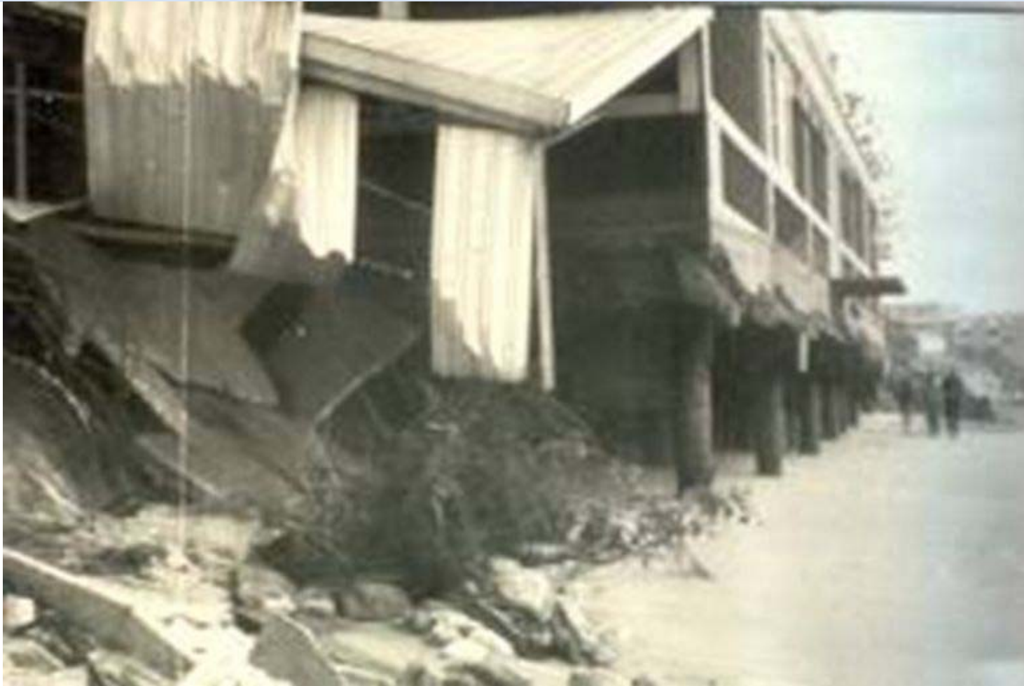
Exposure of 'Flight Deck' foundations as a result of 1967 storms
