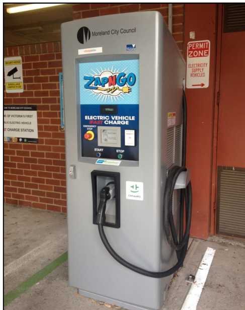
Figure 15 The 'Zap n Go' level 3 fast charging station at Moreland Civic Centre
