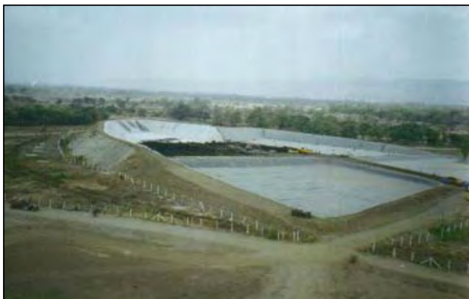
Hazardous waste landfill at Talaja
