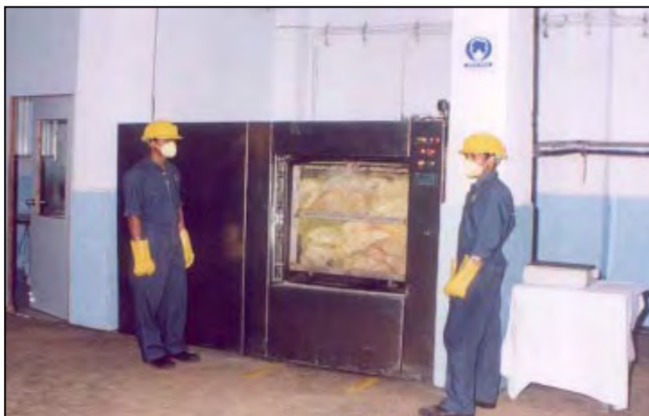
Autoclave at biomedical waste treatment plant
