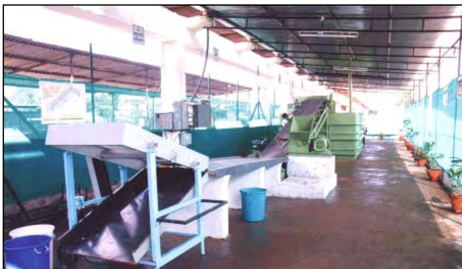
New municipal solid waste treatment unit installed in Pune
