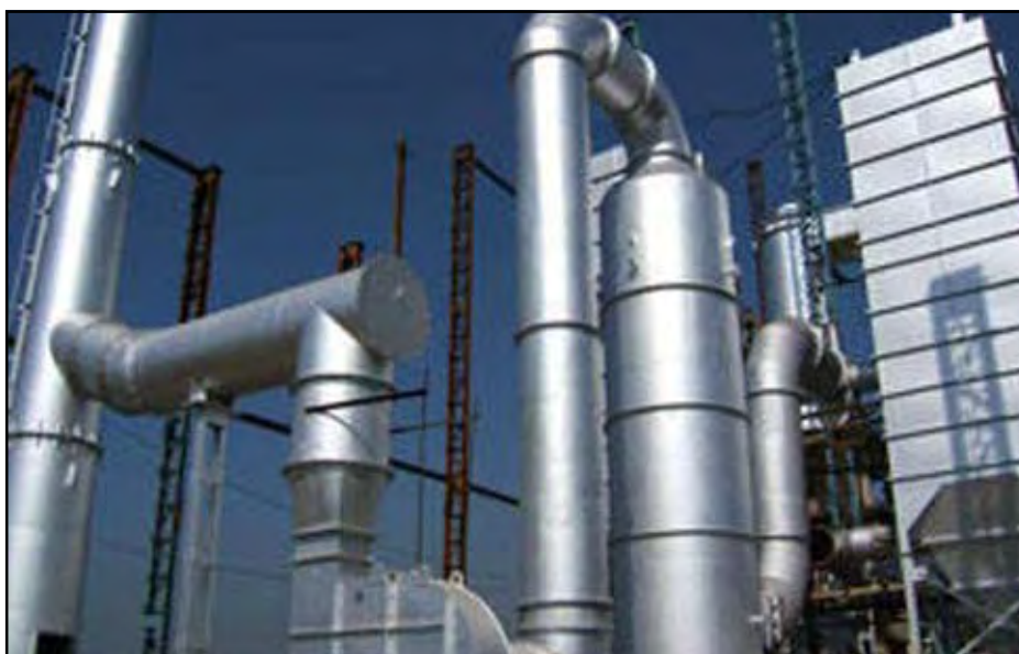
Hazardous waste incinerator at Talaja
