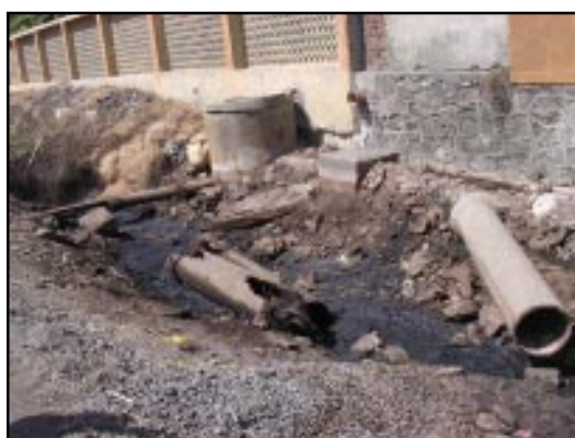
Broken effluent drain at Tarapur industrial estate
