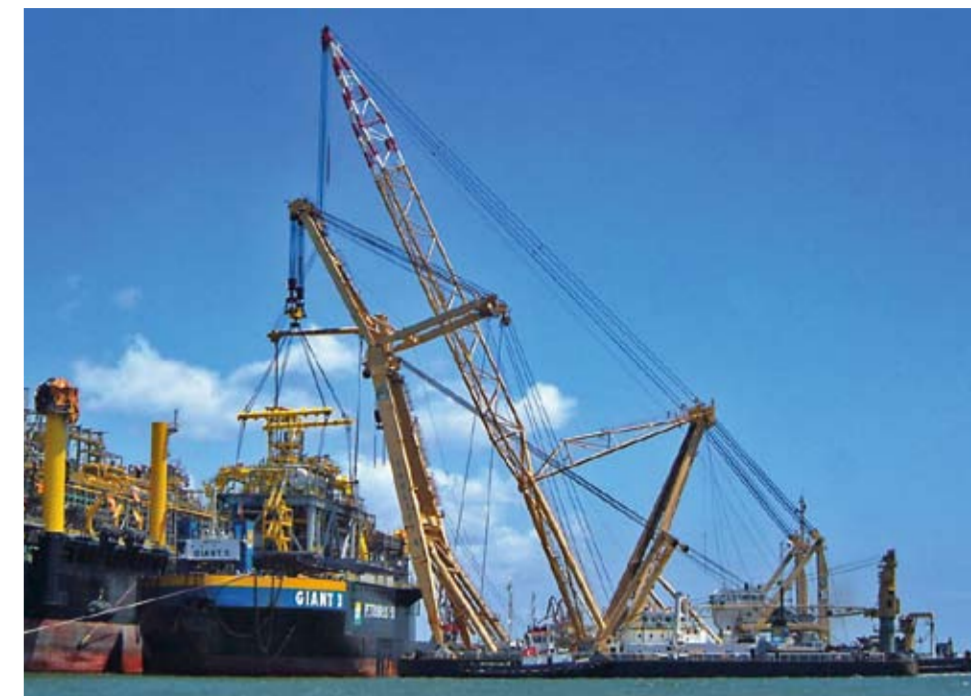
'Giant 3' transported modules for FPU 'P53' from Singapore to Brazil. Sheerlegs 'Takilift 4' and 'Takilift 6' consequently installed the modules onto the FPU.
