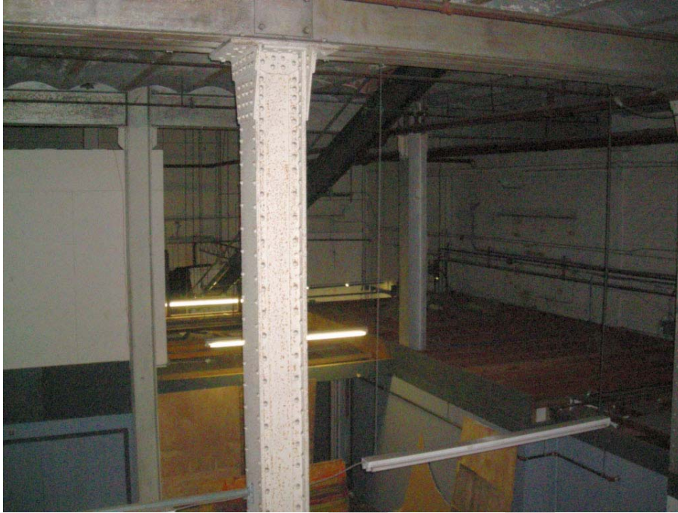
Photograph 11: American Brewing Company building, interior of Engine/Refrigeration House, room 107, showing mezzanine level with main floor level below
