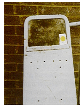
An asbestos cement board on the end of an old ironing board
