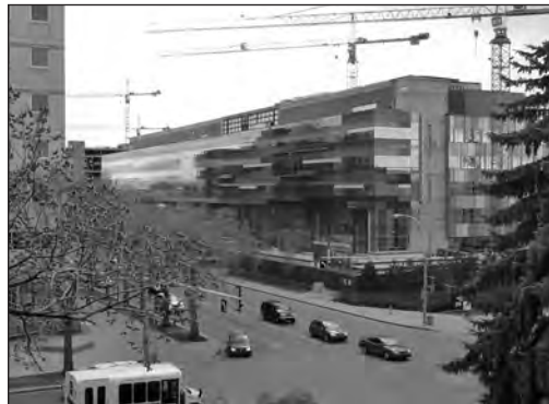
Health Sciences Ambulatory Learning Centre, now known as the Edmonton Clinic North. Construction of Phase I began in 2007.
