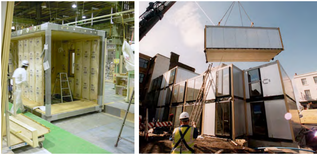
Figure 70 (a) Misawa modular production line near Nagoya, Japan. Photo by James Gardiner (b) Modules being lifted into place for project by Cartwright Pickard Image source - http://www.cartwrightpickard.com/project/live/murray-grove Access date 25th August 2011.
