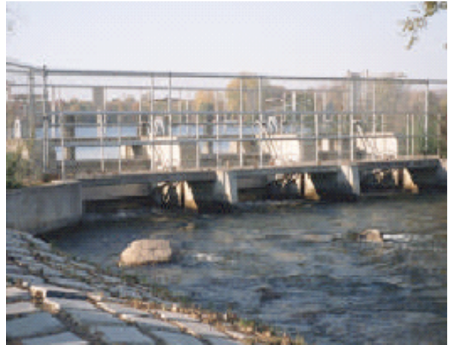
Gray's Bay Dam helps minimize flooding downstream.
