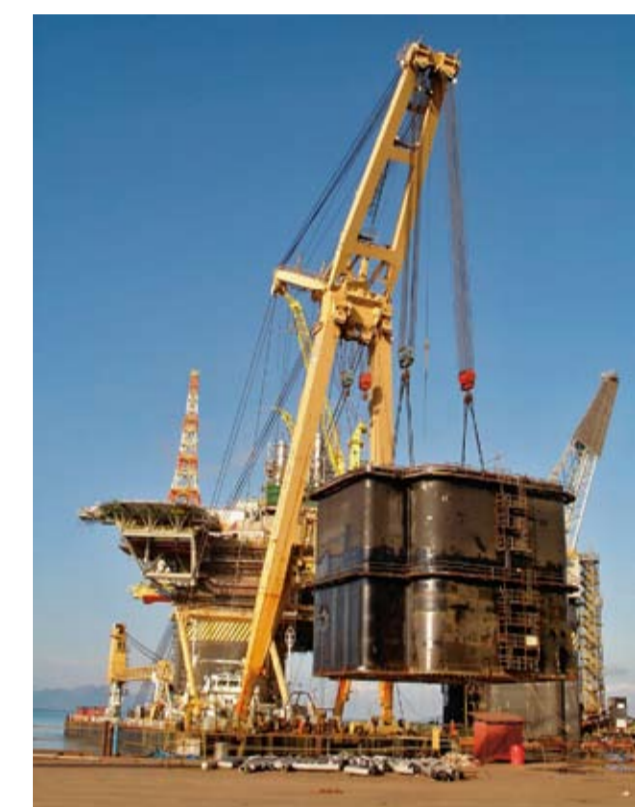
'Taklift 4' during the installation of the fourth column section for the FPU 'P51' in Brasil.
