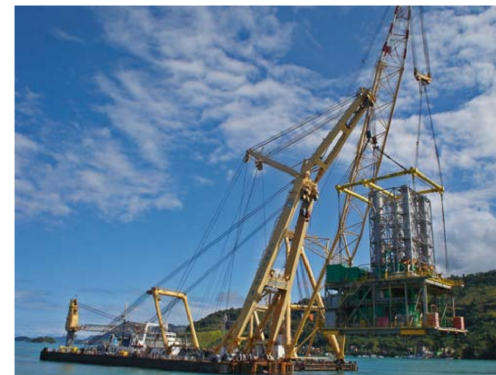
'Taklift 4' and 'Taklift 6' installed several modules for FPU 'P52' in dual lifts in 2006.
