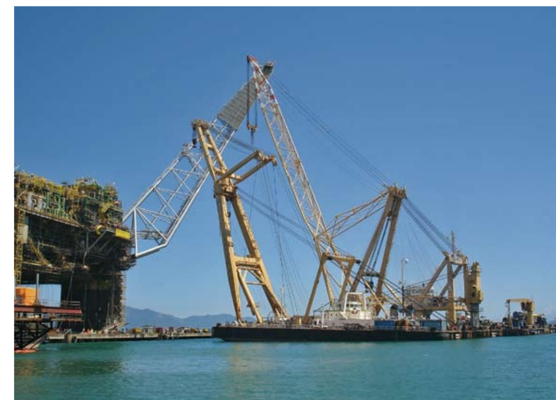
Installation of the flare boom for FPU 'P52' by 'Taklift 4' and 'Taklift 6'.
