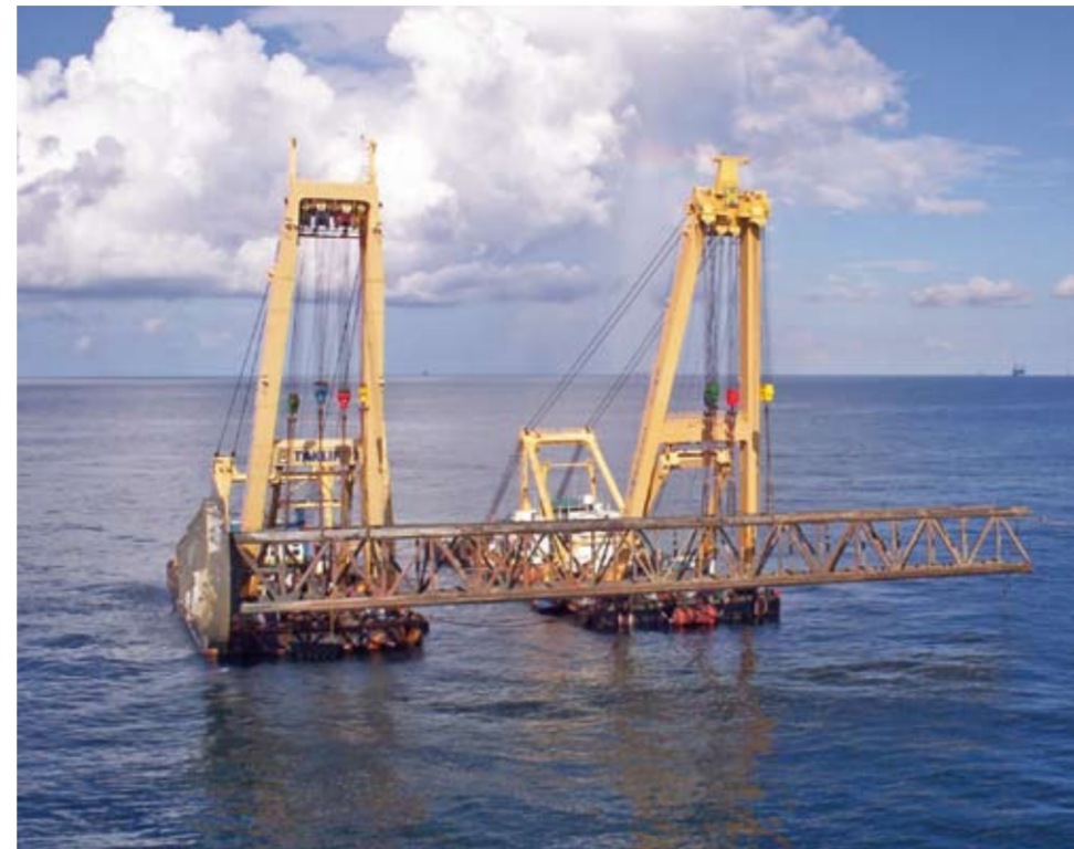
'Taklift 1' and 'Smit Cyclone' removed the legs of the platform 'Ocean Warwick'.
