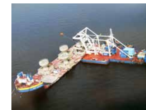
The turbine foundations are offloaded by a heavy lift vessel on site.
