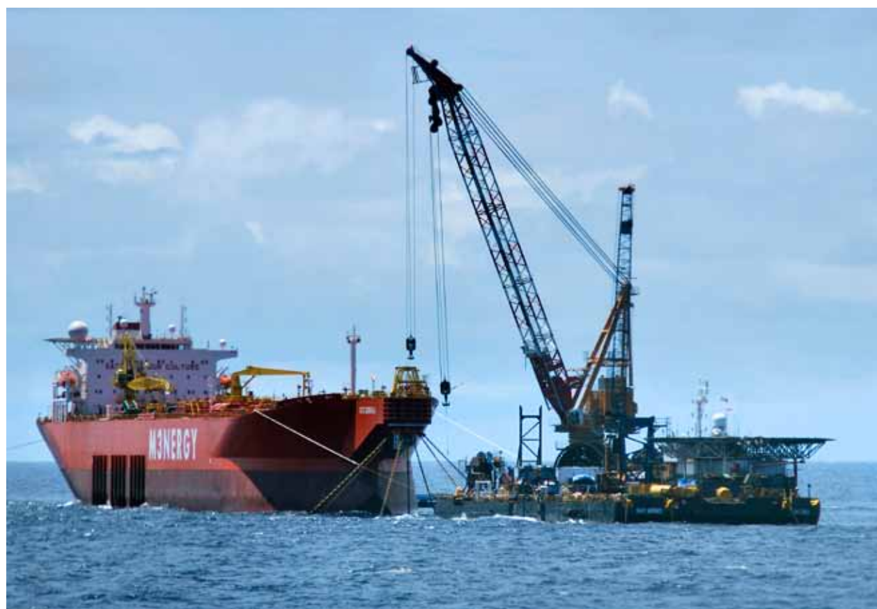
'Smit Borneo' was deployed for the installation of FSO 'Puteri Songkhla' in the Thailand/Malaysia Joint Development Area.
