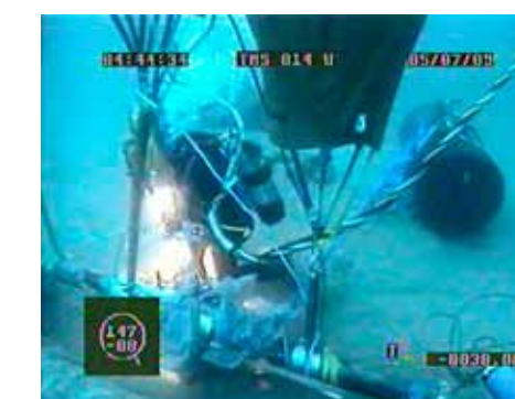
A diver installs the Morgrip pipe connector on to the new pipeline section.
