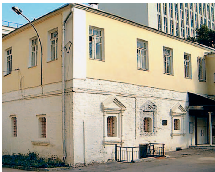
Chambers of the 17th-century Pharmacy Directorate in Starovagankovsky Pereulok, Moscow. The second floor was added in the 1920s
