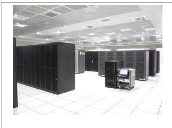
Figure-10: ISSDC Computer Server Room
