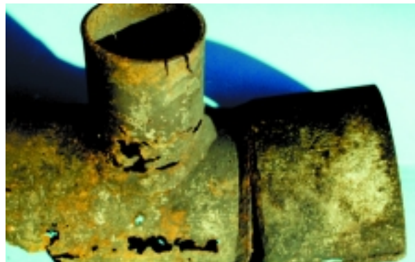
Top: Tube fouling in an incinerator plant due to carryover of deposits.
