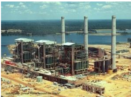
Figure 40. Martin Lake station
