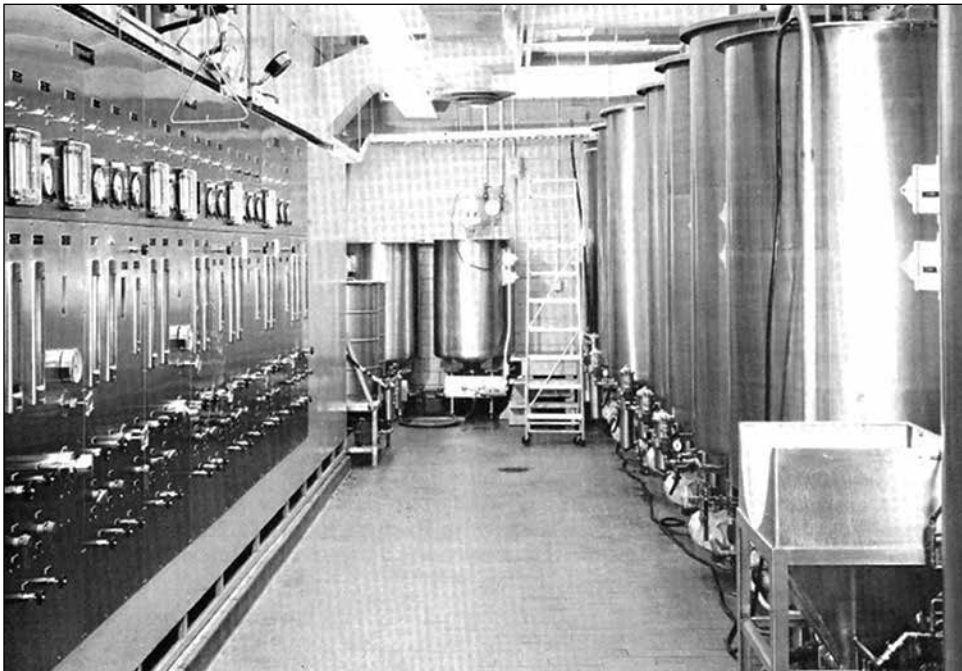
Figure 24: Bridgehead B&W Chemical Mix and Storage Room with Distribution and Replenishment Panels at Left. Ground Handling Equipment for Reconnaissance/ Aerial Photography Fact Sheet, July 1977, produced by Bridgehead's Special Programs unit.
