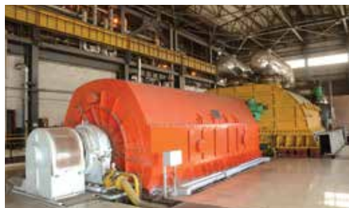
Turbine at BALCO power plant
