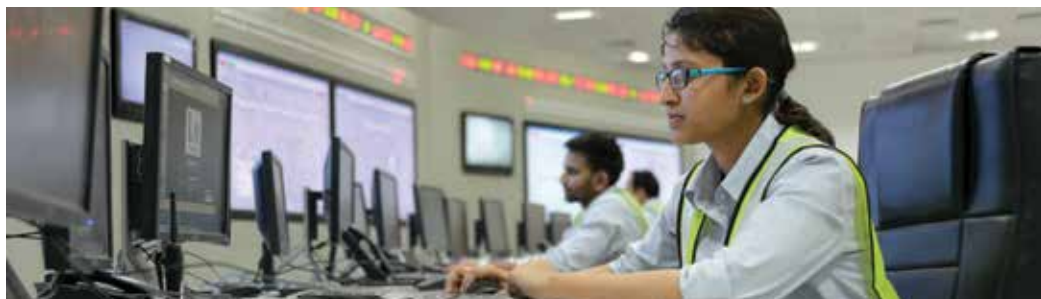
DCS- Control Room, Vedanta Limited - Lanjigarh
