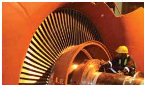
Turbine generator, Talwandi Sabo
