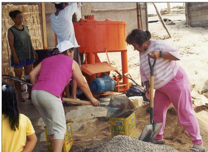
Figure 5. Women producing concrete blocks and other types of cheap building materials for self-help housing when upgrading poor settlements in Lima, Peru, under the guidance of barefoot architects and engineers within Non-Government Organisations such as Estrategia and ARC•PEACE Peru. (Photo: Luz Maria Sanchez).
