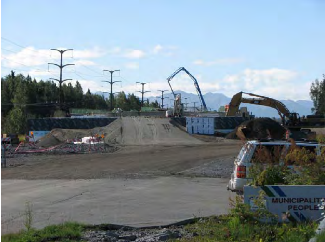
Fig. 88 – Bragaw St. Extension over Campbell Creek near the Municipal Offices, August 2007 (photo by author)
