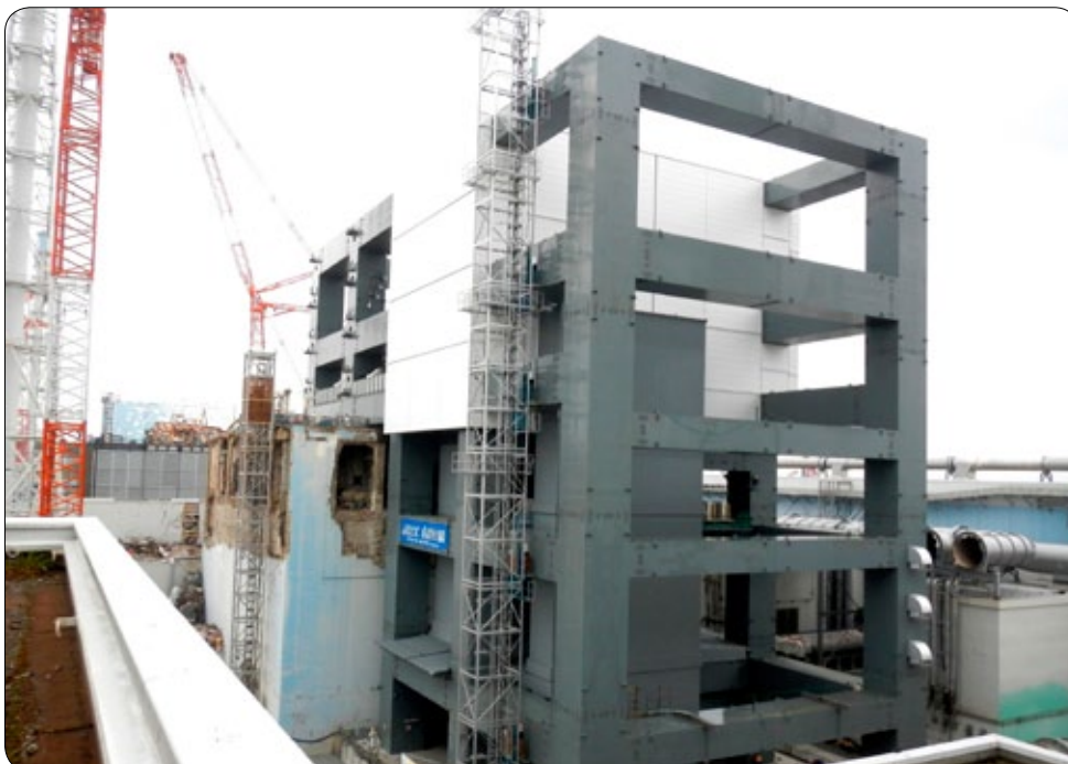
Steel frame for fuel removal at Unit 4 of Fukushima Daiichi Nuclear Power Station
