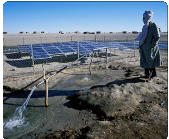
Solar Voltaic used to pump water out the ground, Oasis Salal, Bahr el Ghazal, Chad
