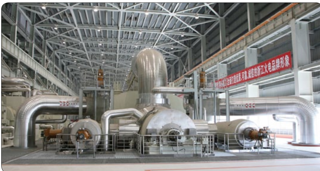
Modern ‘ultra supercritical’ technology raises efficiency in coal-fired power plants
