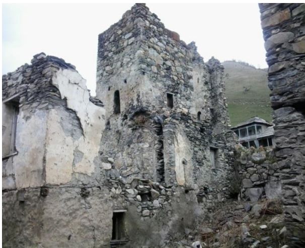
Photo 5.4.2. Collapsed Machubi and tower in Hadishi
