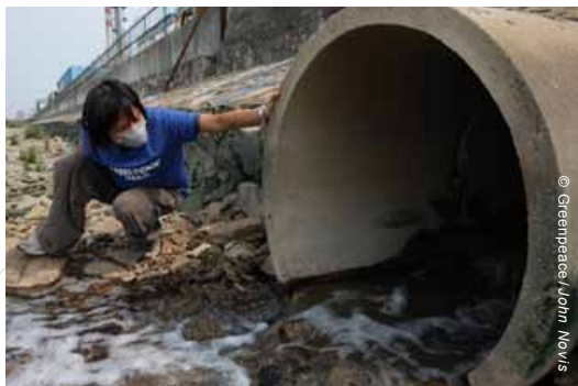
A discharge outfall connected to the outside wall of the industrial area
