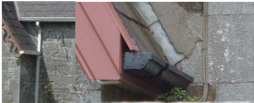
White uPVC guttering and drainage (left) replacing original black cast iron (right)
