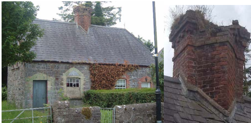
Stone houses 7 (left) and 8, and the shared chimney, in need of repair
