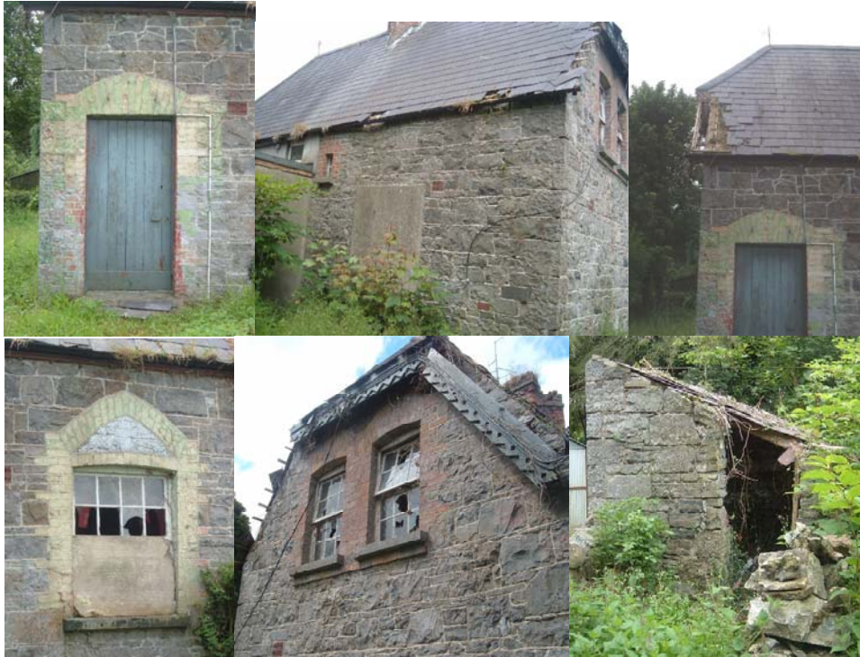
House 7, showing the damaged brick detail surrounding the doorway, problems with the roof, guttering, broken windows, damaged fascias and the shed.
