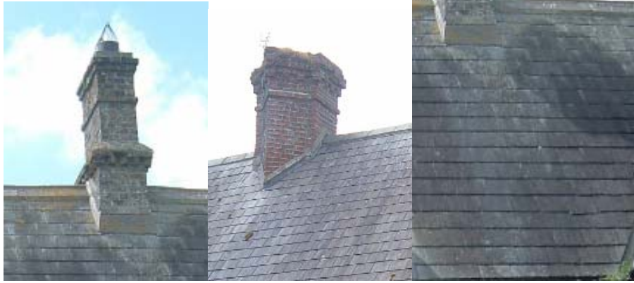
Traditional brick chimneys and slate roofs. The ridge tiles are also original.
