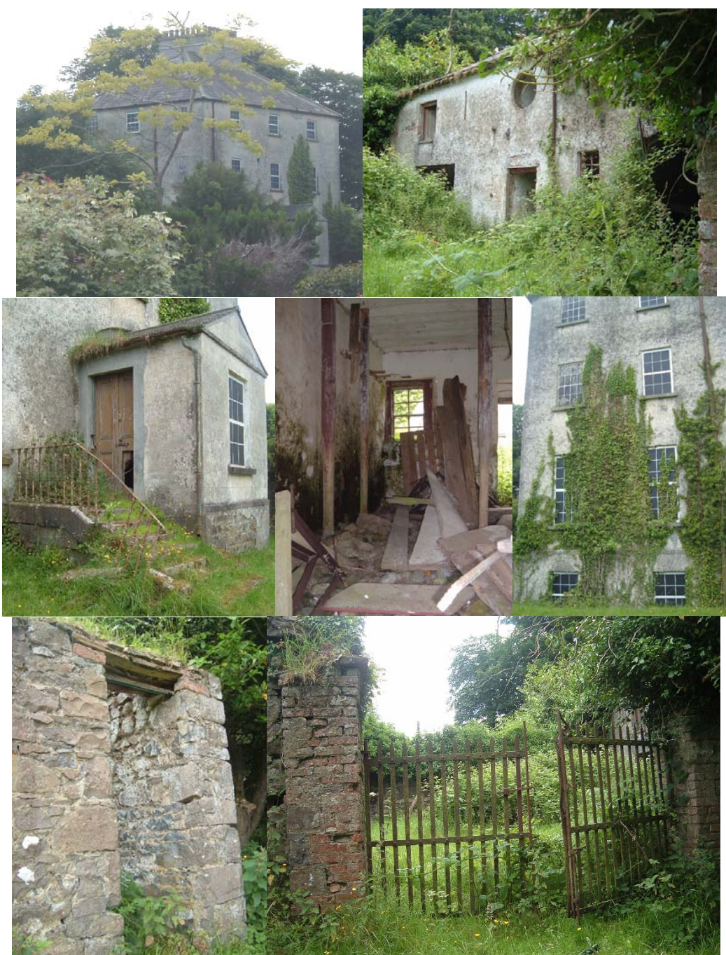
Glebe House (Rectory) from the road, built in 1823, uninhabited since the 1960s (top left), the outbuildings (top right), the main entrance to the house (middle left) inside the outbuildings (centre) the extent of the ivy growth, and one of the cast iron drainpipes (middle right) a seriously weathered outbuilding (bottom left) and the gates leading into the rear of the rectory/outbuildings complex (bottom right).
