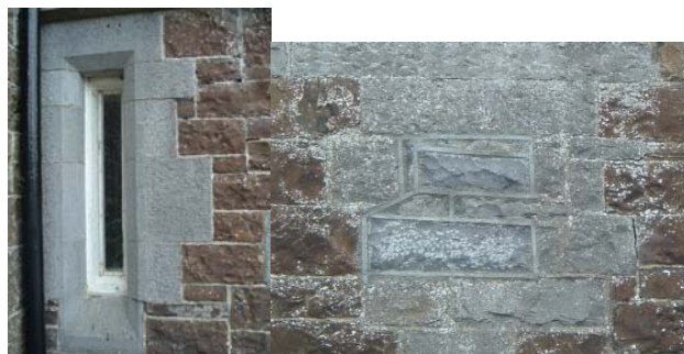
One of the narrow windows in the porch, and a mark showing repairs where an insignia once was but has been removed, above the door.
