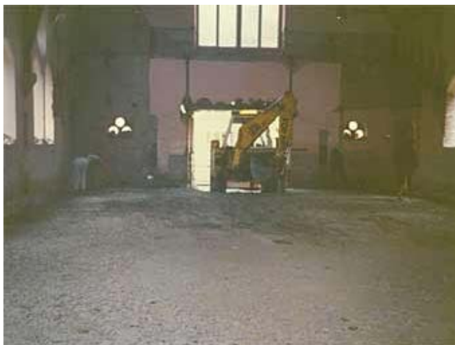
After the pews had been removed, the big machines moved in to excavate the ground floor.
