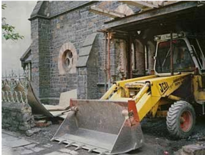
← An opening large enough for a JCB machine was created in the front wall of the building. →
