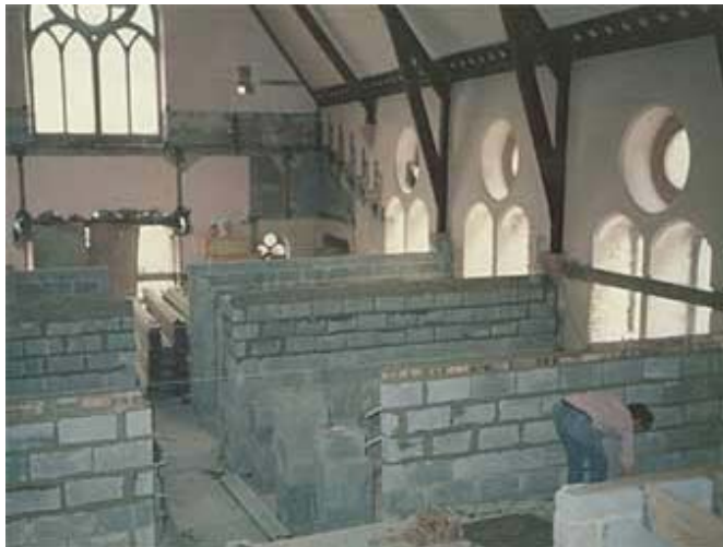
Internal walls were built to create consulting rooms and other areas for the new doctors' surgery.
