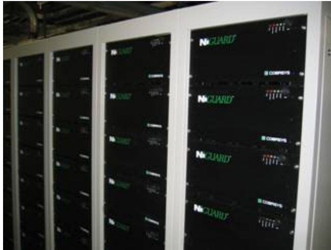
Figure 7. Chevron Bellaire Center with Cobasys NiMH Batteries
