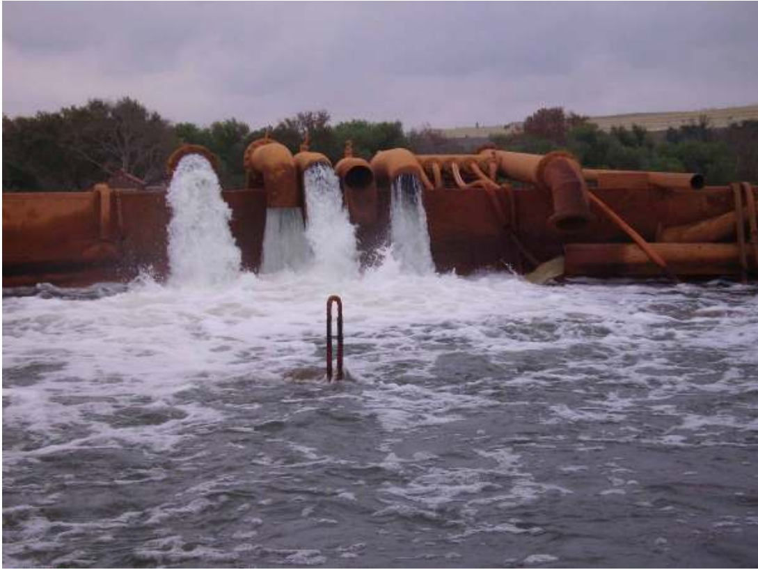
Figure 4.4. Water pumped from the Eastern Basin to the treatment plant at Grootvlei Mine
