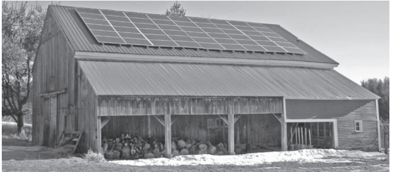
This solar installation on a barn in Gorham generates power for the owner's early 19th century farm. Landmarks can provide advice for homeowners considering solar photo-voltaic power in historic contexts.
