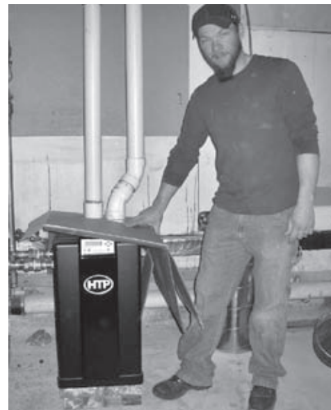
Safford House will use less energy thanks to a high-efficiency, state-of-the-art boiler, shown by Jason Le Shane of Wright-Ryan Construction.
