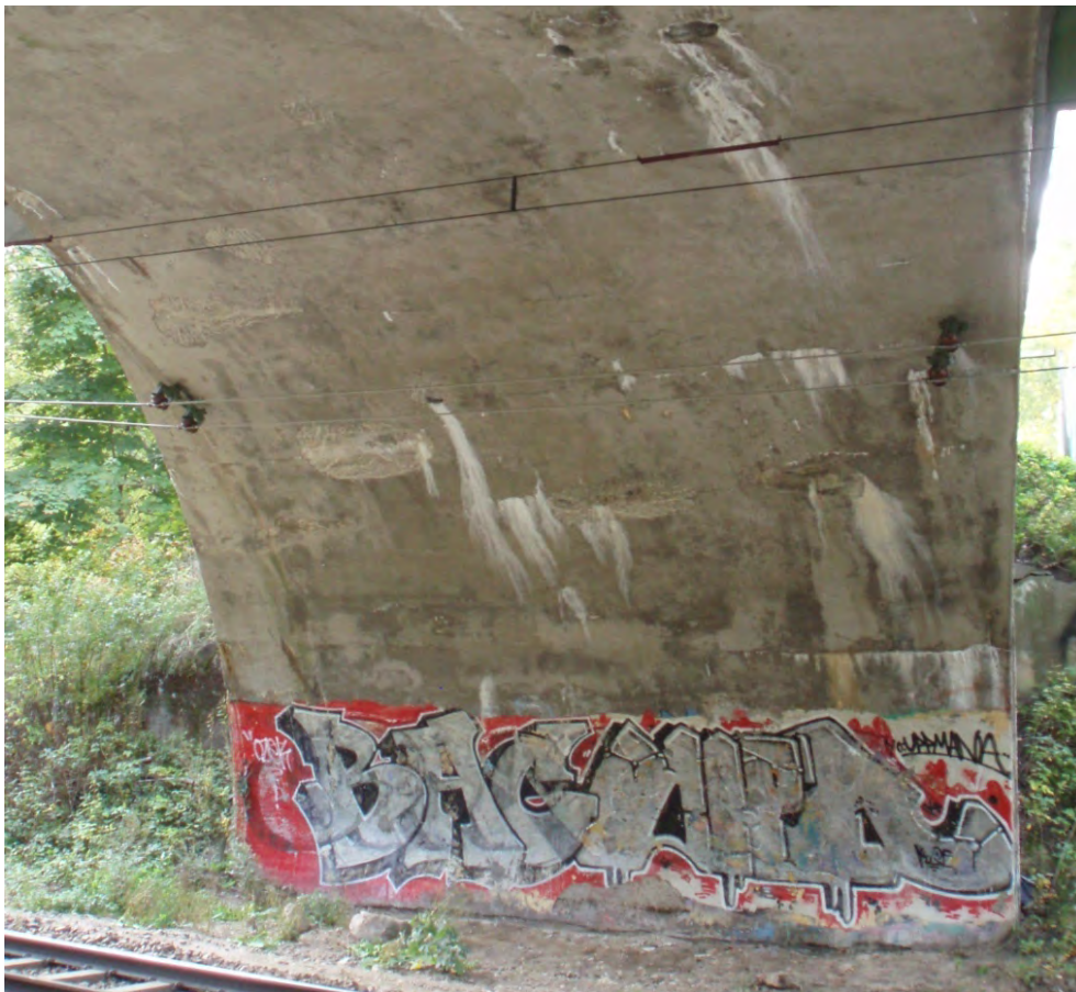
Figure 3.11: The leakage is seen as white marks on the concrete.
