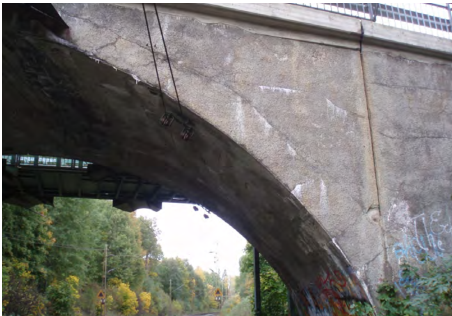
Figure 3.9: Crack between the arch barrel and the spandrel.
