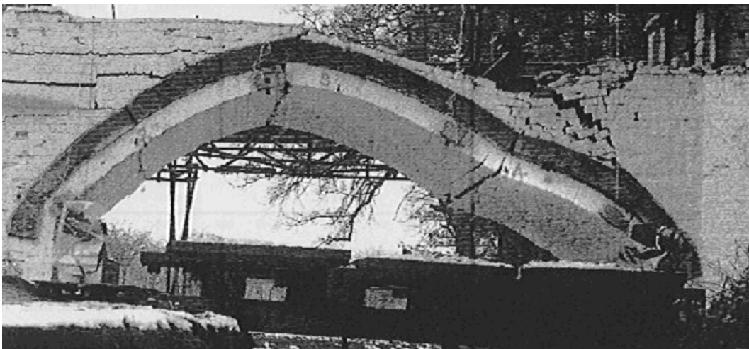
Figure 2.2: The Prestwood Bridge during failure at the haunch, (Sowden, 1990).
