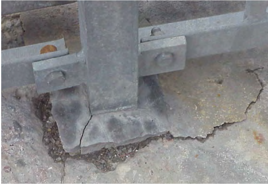
Figure 3.8: Cracks in the edge beam caused by frost erosion.
