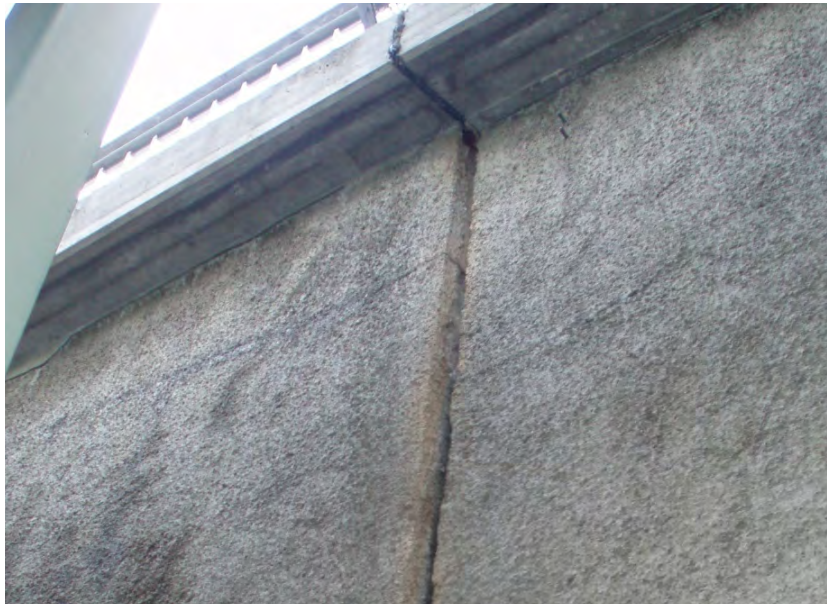
Figure 3.7: The joint between the spandrel and the side wall of the abutment.
